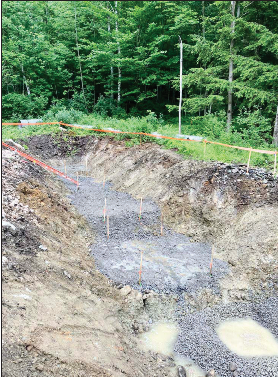
Excavation began immediately for the new dam's foundation, anchored in bedrock beneath the Pond's outlet. The solid concrete structure will be 250 feet wide to meet the latest safety standards, deepen the Pond and put an end to its fluctuating water levels. (Bob Low photo)
