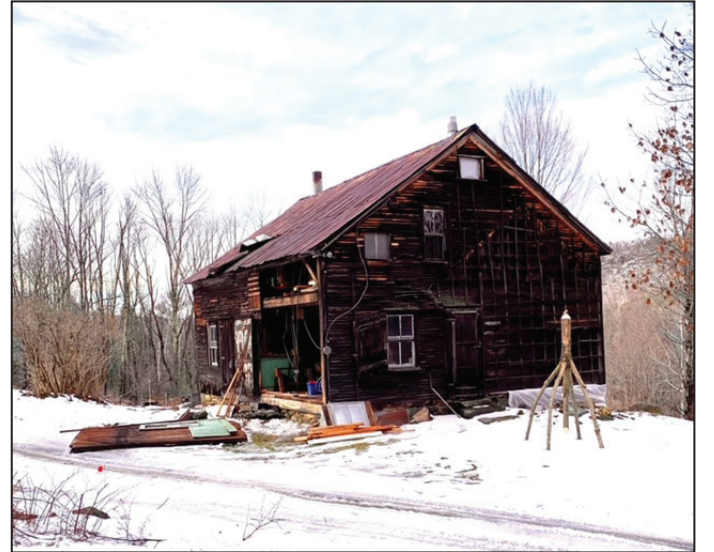
Old farmhouse, now used for storage by Duncan and Megs Keir, had most of a side blown off during recent high winds in Huntington. The Keirs also lost shingles from the roof of their new house. Courtesy photo
