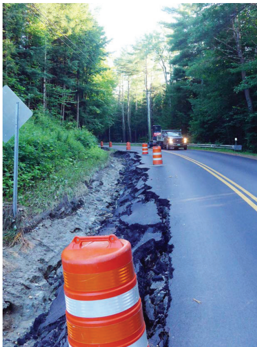
July damage to Huntington Road's Richmond Hill from culvert damage and ditch flooding reduced the road to one lane as the crew scrambled to do repairs. Truckloads of gravel and sediment washed down the hill and were dumped into the field near the intersection with Hinesburg Road. Photo: Bob Low
