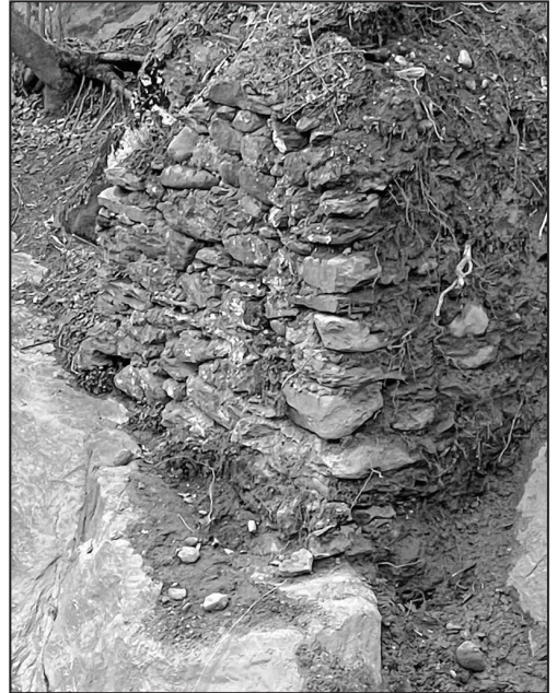
An old, stone abutment shows itself from the vantage point created by the washout on Dugway Road.
